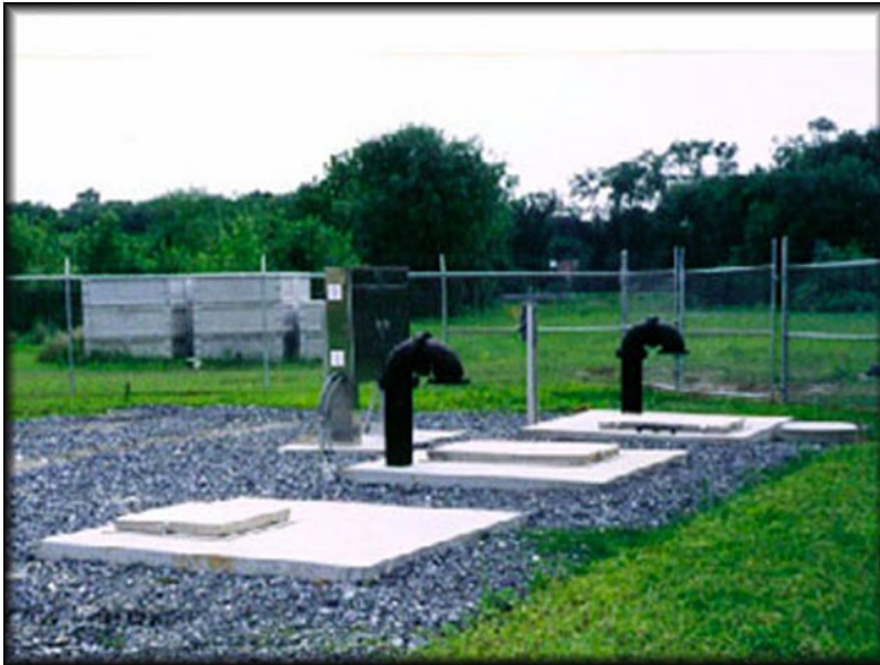
6 foot pump station
