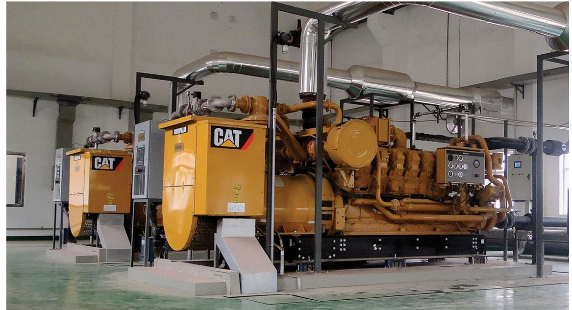
1,000kW Generator, Caterpillar
