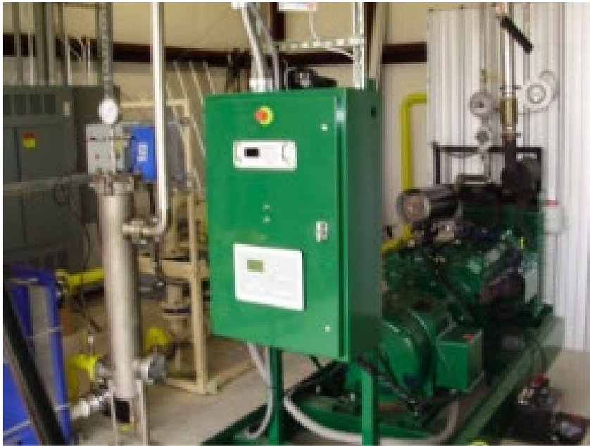
75kW Generator, Ford 460C.I. V-8 Montgomery Regional Solid Waste Authority (MRSWA) in Christiansburg, Virginia
